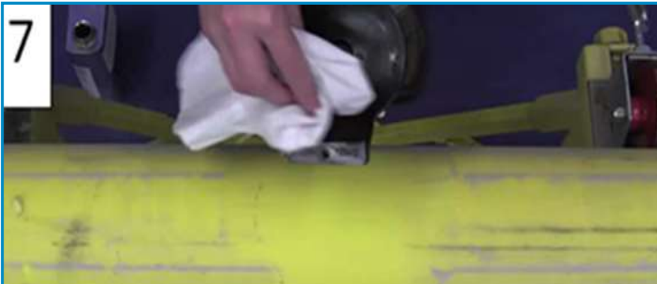
7 Often, the same cloth is used to clean the PE pipe and electrofusion saddle fitting
