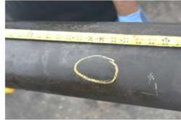
(a) Joint 2 (20.1'-60.6') showing little corrosion
