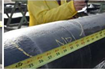
(b) Joint 14 (517.8'-560.4') showing shallow corrosion
